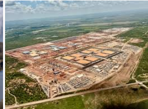
$500B U.S. backed 'Stargate' data center initiative
